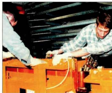
Nearly 80 new magnets were installed in the HERA tunnel for the upgrade in 2000/2001 to enable a higher luminosity.
